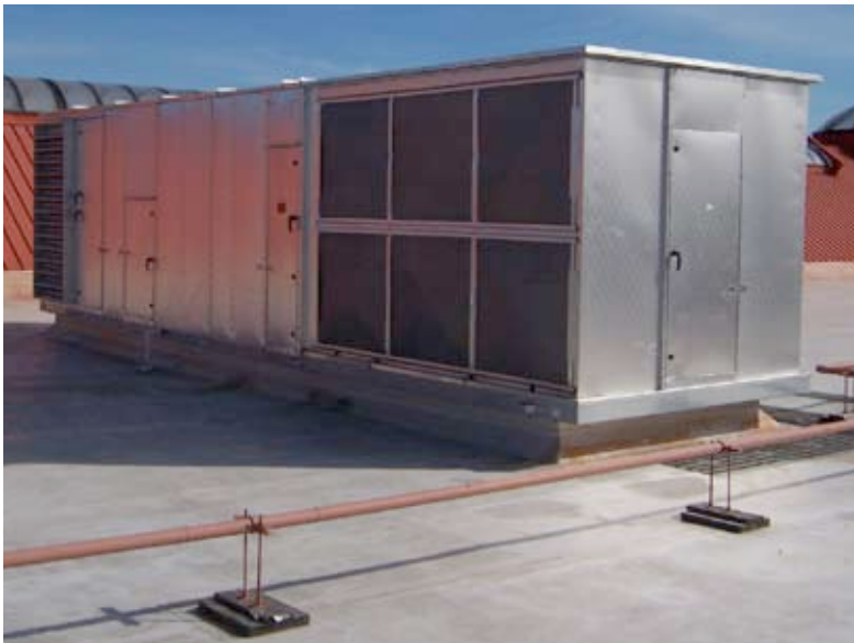
This rooftop boxcar replacement for Pheasant Lane Mall in Nashua, NH, was custom manufactured to fit on exactly the same roof curb as the previous unit to minimize roof work required. As a result, the unit was up and running the next day.
